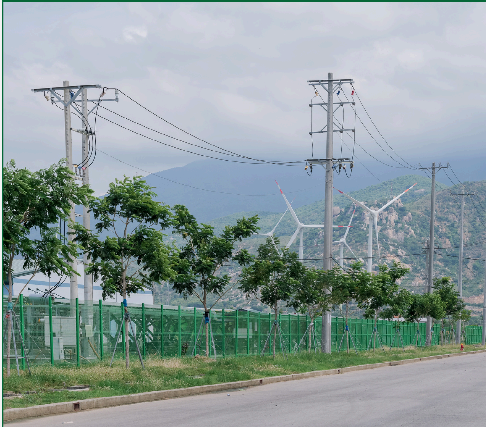
Power source - electricity supply
