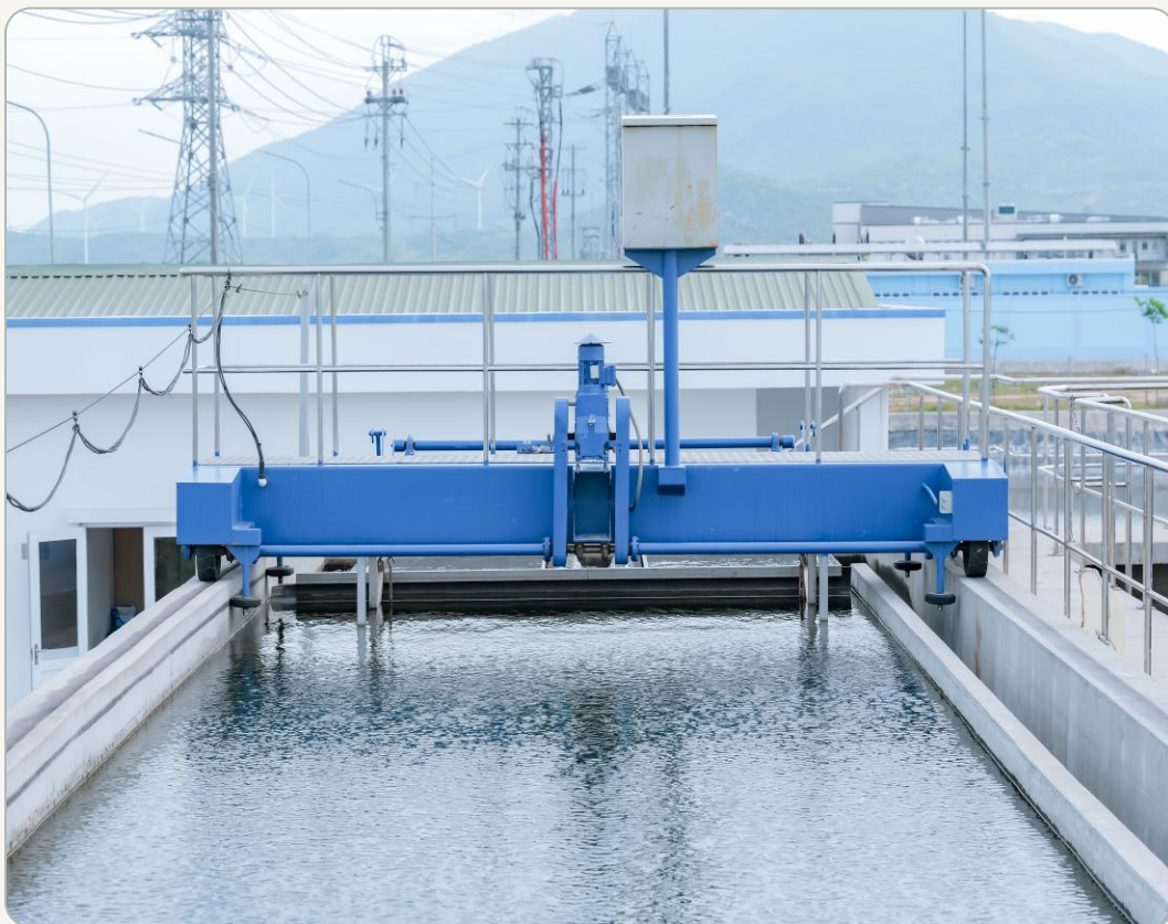
Wastewater-treatment plant image – Module 01
